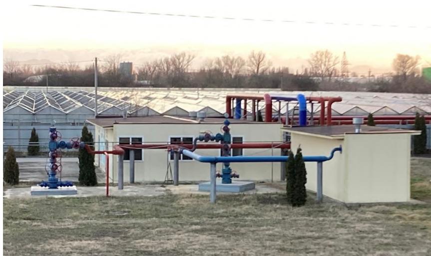
Fig. 3. Pilot industrial geothermal plant based on the implementation of a circulation scheme for the use of deep Earth heat. Khankalskoye thermal water deposit.
