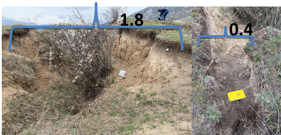
Fig. 2. Cracks (joints) observed in the landslide site of the Hovq settlement
